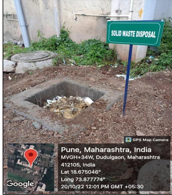
Solid waste disposal by compost pit
